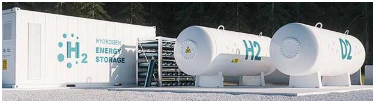
Small-scale hydrogen storage tanks (source: link )
