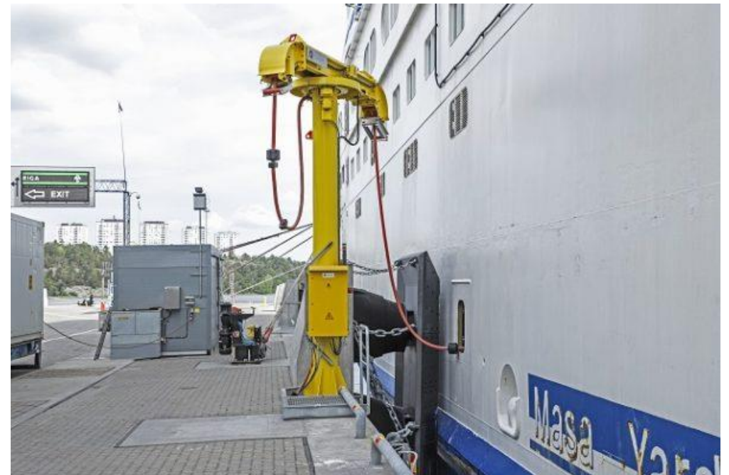
Cold ironing machinery in the port of Stockholm 2
