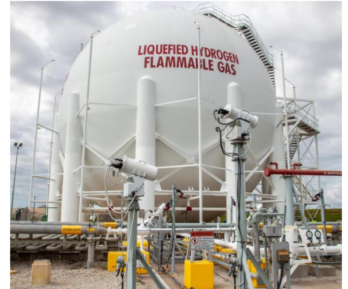
Liquid hydrogen Tank at NASA Kennedy Space Center (source: link )
